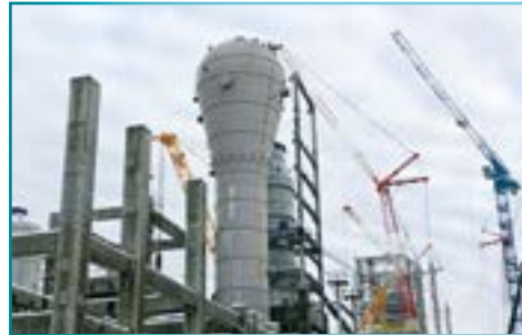
Gas-phase polymerization Technology Product 2 units Innovene G HDPE/LLDPE
